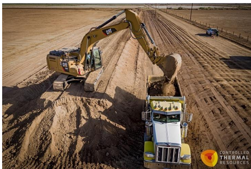
Construction begins on the Hell's Kitchen Geothermal Project (photo courtesy of Controlled Thermal Resources)
