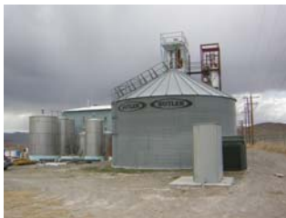
The grain silo, methanol recovery towers, and the tank farm at the Wabuska bio-diesel facility; under construction. Photo by Claude Sapp, Infinifuel Biodiesel: http://www.infinifuel.com/ Used by permission
